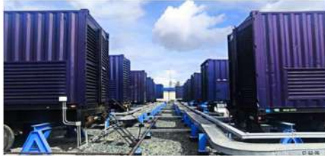
Array of containerized MGS2500R that powers Bohol during power outages.
